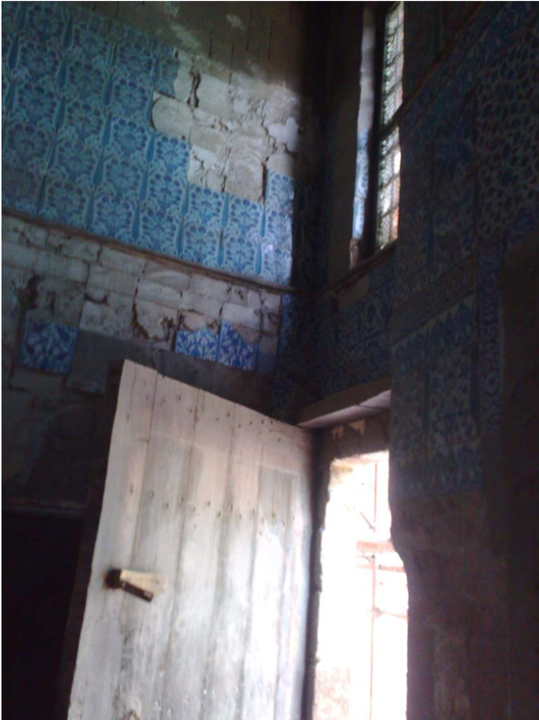
Picture A4: Bulging Mausoleum walls and cracked and fallen ceramic tiles.
