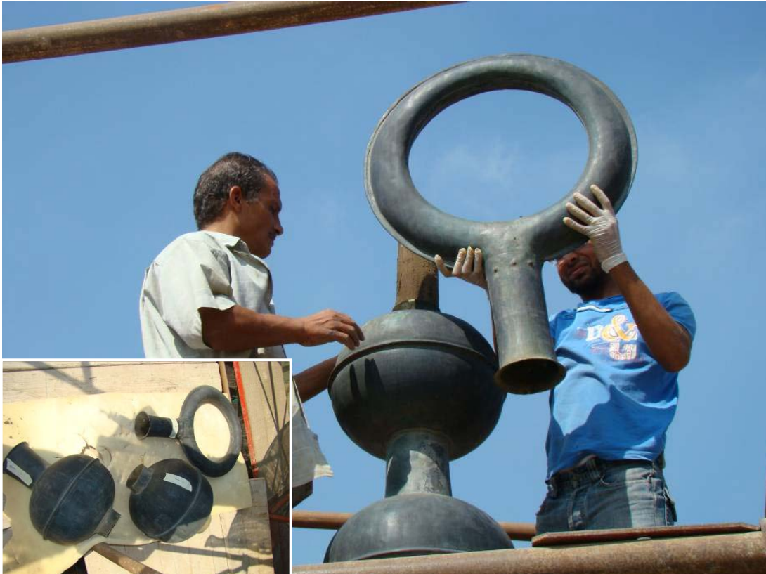
Dismantling and numbering of the brass crescent to enable the replacement of the led sheets
