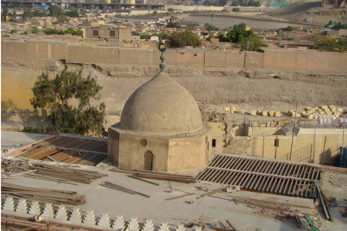
General view of SE roof after placing the steel I-beam and completing the carpentry activity
