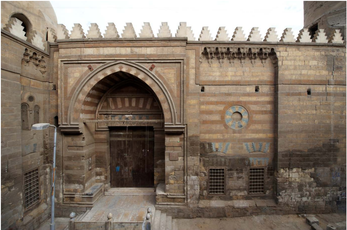
(Top) The Mosque's entrance portal and main façade lining Darb al Ahmar Street. The general damage pattern of the Mosque's elevations is marked by a line of salt migration from the ground up to 2-3 m, creating decay to the stone veneer (desquamation) and on the mortar joints (powdering). Cause of this moisture damage appears to be a combination of the Cairene habit of watering the streets, garbage deposits at the foot of the facades and leakage of the underground main potable water pipes.
