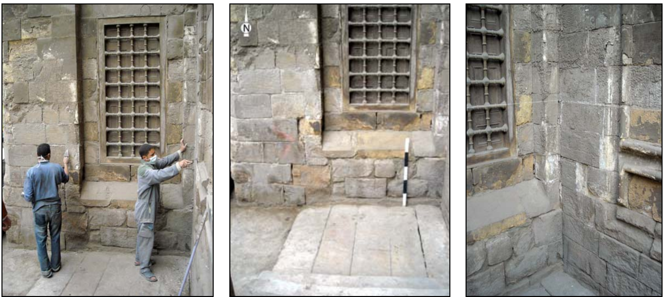
doc. 5a : Cleaning the façade of the mausoleum / 5b : after cleaning / 5c : Junction between the two ensembles.
