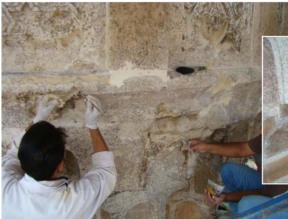
Re-pointing of joints and mortar completion of cracked and eroded stone parts
