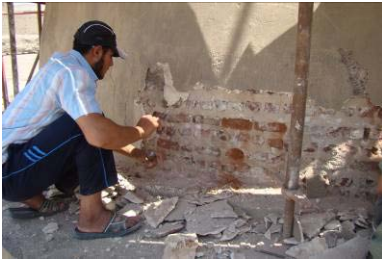
Flaking the plaster
