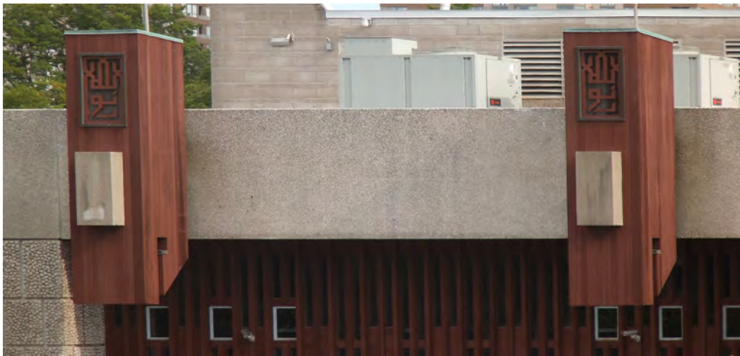
FIGURE 5.11 Exterior lantern (detail). Moriyama & Teshima Architects, Noor Cultural Centre, Toronto, Ontario, Canada. Originally built, 1963. Purchased in 2005. Photo: Nadia Kurd, 2013.
