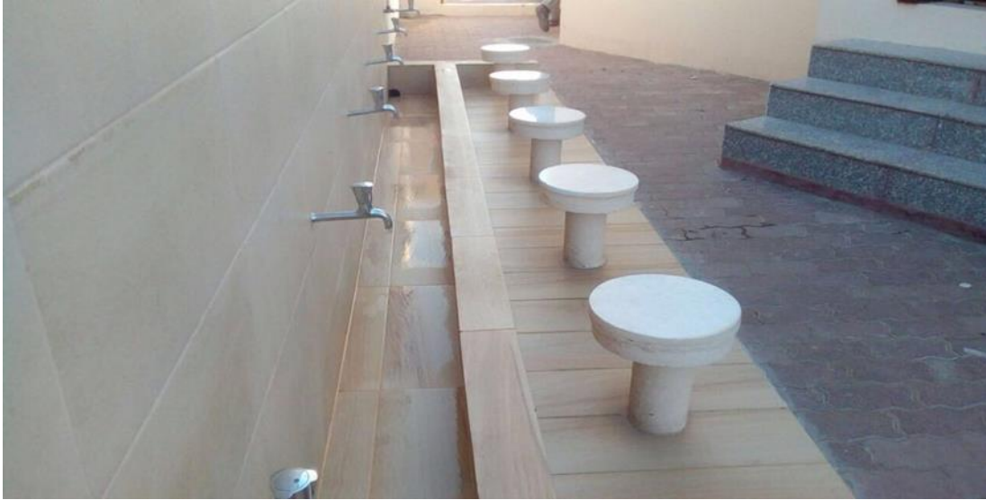
Figure 4.7: Normal taps controlled by users for opening and closing in the fifth mosque
