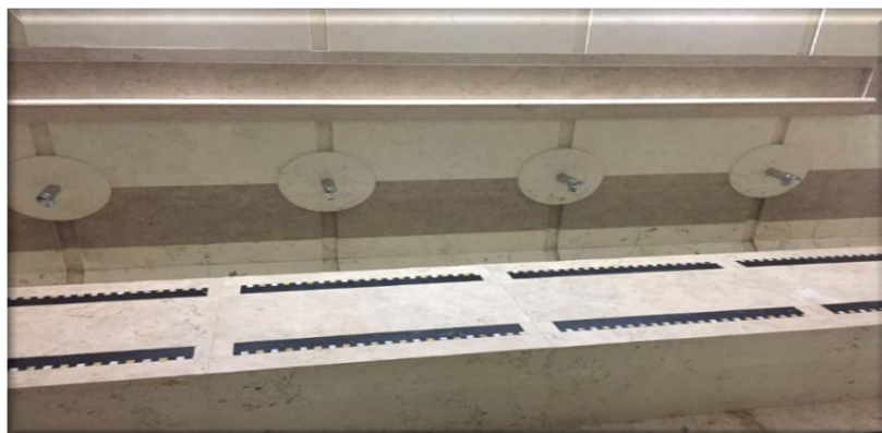
Figure 4.1: Push taps controlled by a timer in the first mosque (Jame)
