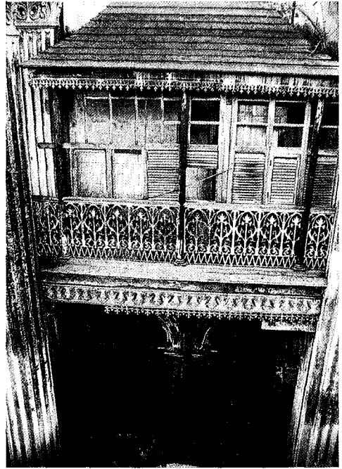
Balconies at Ruplal House, presently used as toilets.
