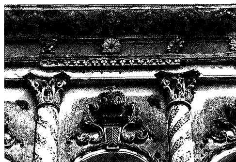
A close-up of Building 32, Kashinath Bhaban, shows that the surface of the columns is striped with broken china pieces
