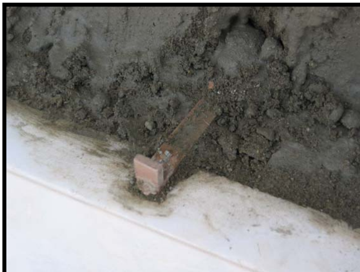
Gun metal clamps were used to anchor the marble slabs to the brick wall.
