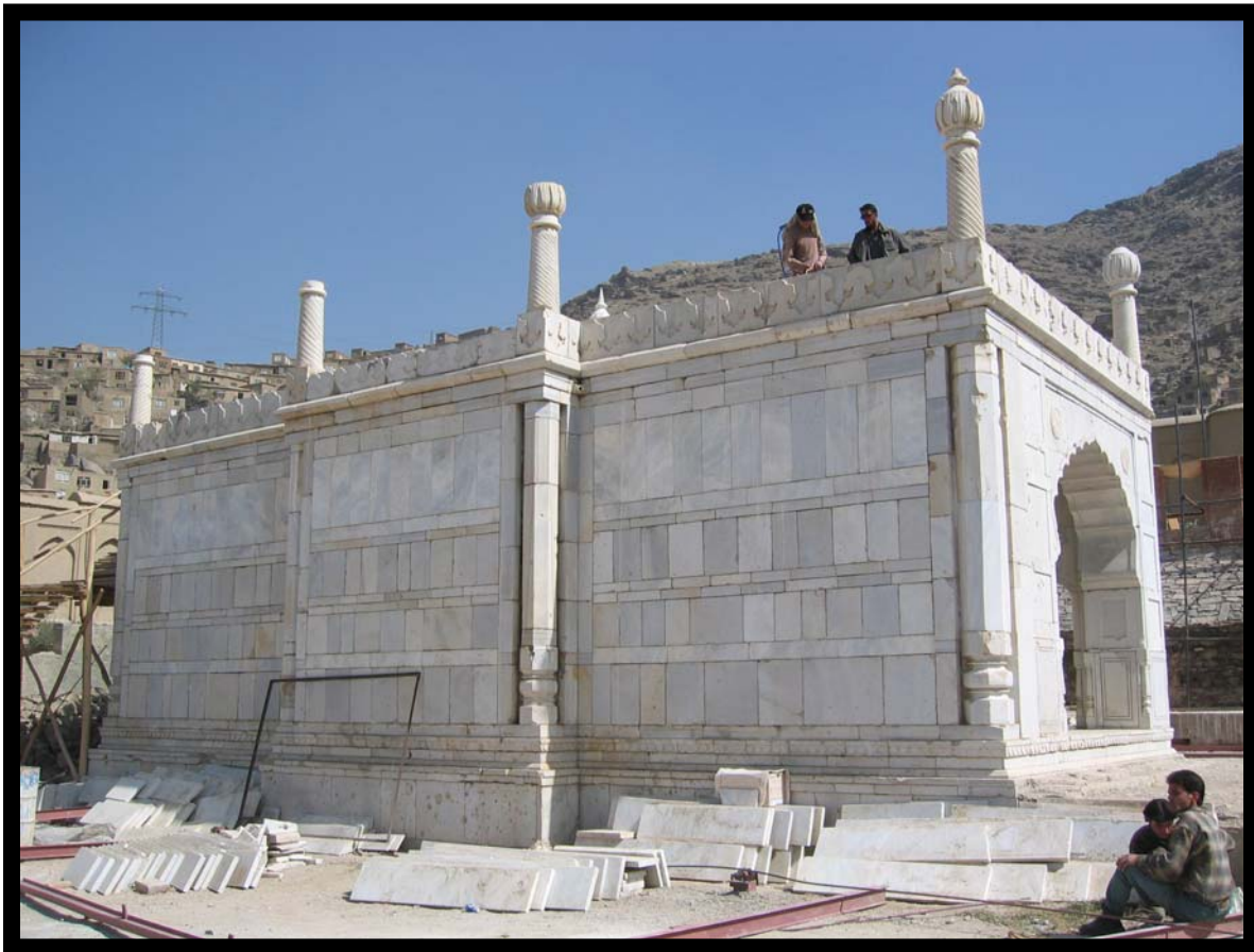
The west wall after the completion of the marble facing, repair of the parapet and removal of the temporary roofing. Marble slabs on ground are for the paving.
