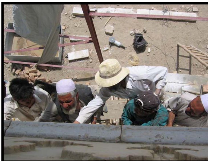
The marble craftsmen, master mason and assistant labour fixing the top marble row.
