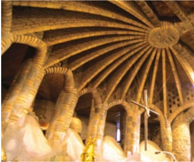
Fig. 7 Gaudi's buildings show that personal creativity and new architectural shapes are not at odds with using traditional techniques. Cripta Colonia Güell vault, Barcelona, Spain (photo: F. Vegas, C. Mileto).
