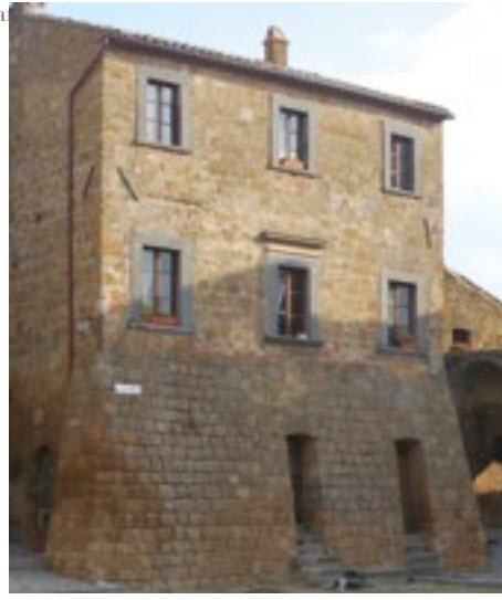
Fig. 2 Reinforcing all the ground floor at Civita di Bagnoregio, Lazio, Italy (photo: S. Onnis).
