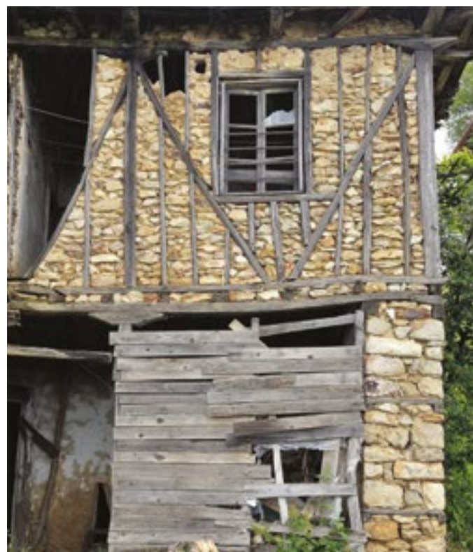
Fig. 16 House with a stone-built ground floor and a wooden frame structures with stones infill in the region of Gotse Delchev, Bulgaria (photo: S. Mecca).
