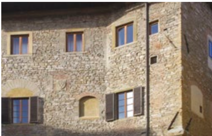
Fig. 4 Anchor plates in a stone building in Florence, Italy (photo: L. Dipasquale).
