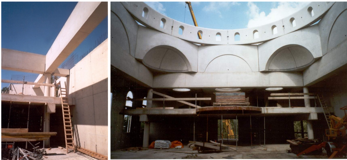
Fig. 12 and 13. The construction of the dome's structure made of prefab concrete elements. Source: (Toorman Architecture Archive, 2021)
