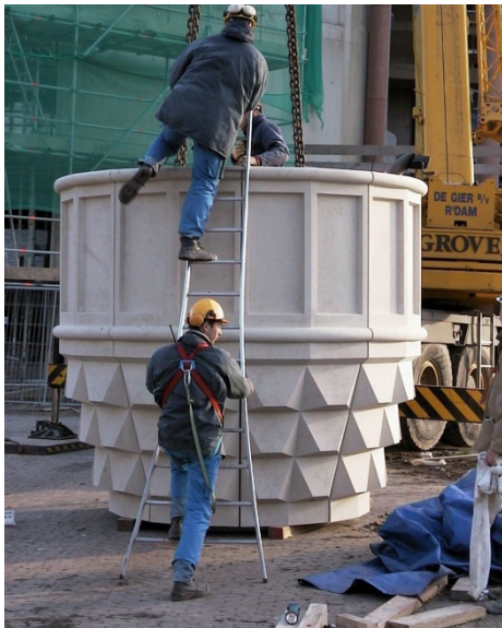
Fig. 24. Prefab concrete structure for the balconies of the minaret. Source: (Toorman Architecture Archive, 2021)
