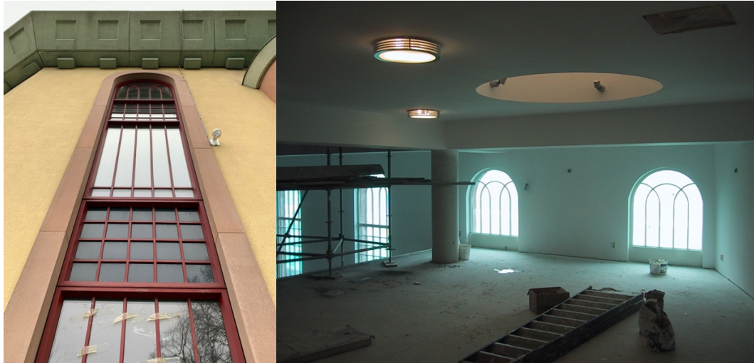
Fig. 30 and 31. Plastic window frames used for façade openings due to financial reasons. Source: (Toorman Architecture Archive, 2021)
