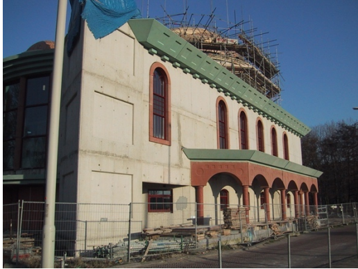
Fig. 22. Concrete used for the structure of the mosque. Source: (Toorman Architecture Archive, 2021)
