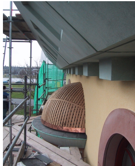
Fig. 25. Wooden structure used for substructure for the patinated copper domes. Source: (Toorman Architecture Archive, 2021)
