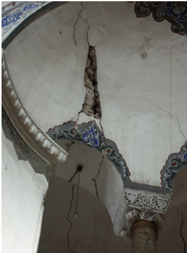
Figure 7 Interior damages one of the small domes next to the main dome
