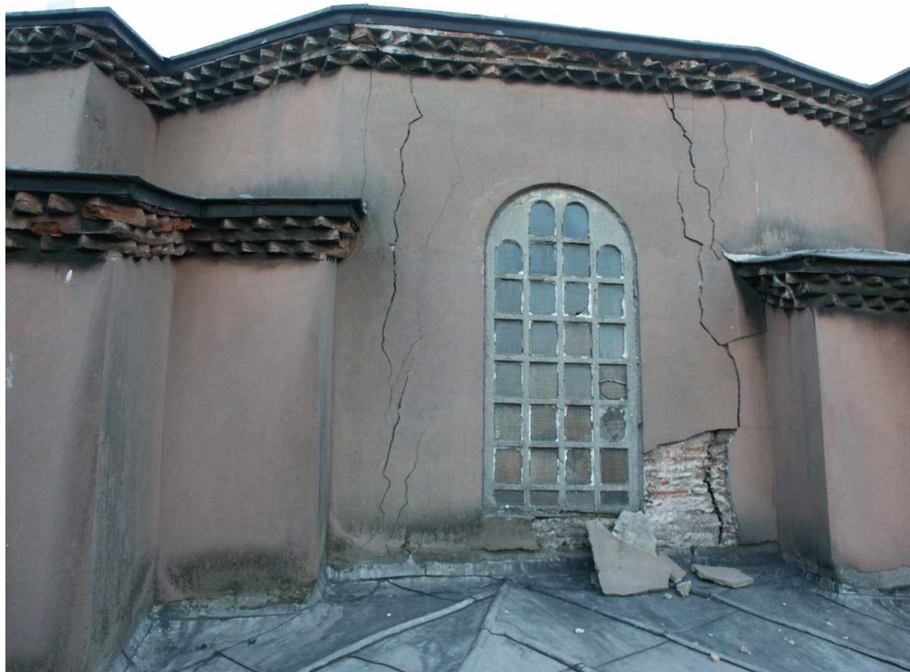
Figure 8 Crack patterns of the periphery wall of the main dome
