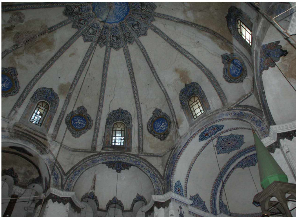
Figure 9 Interior cracks of the main dome
